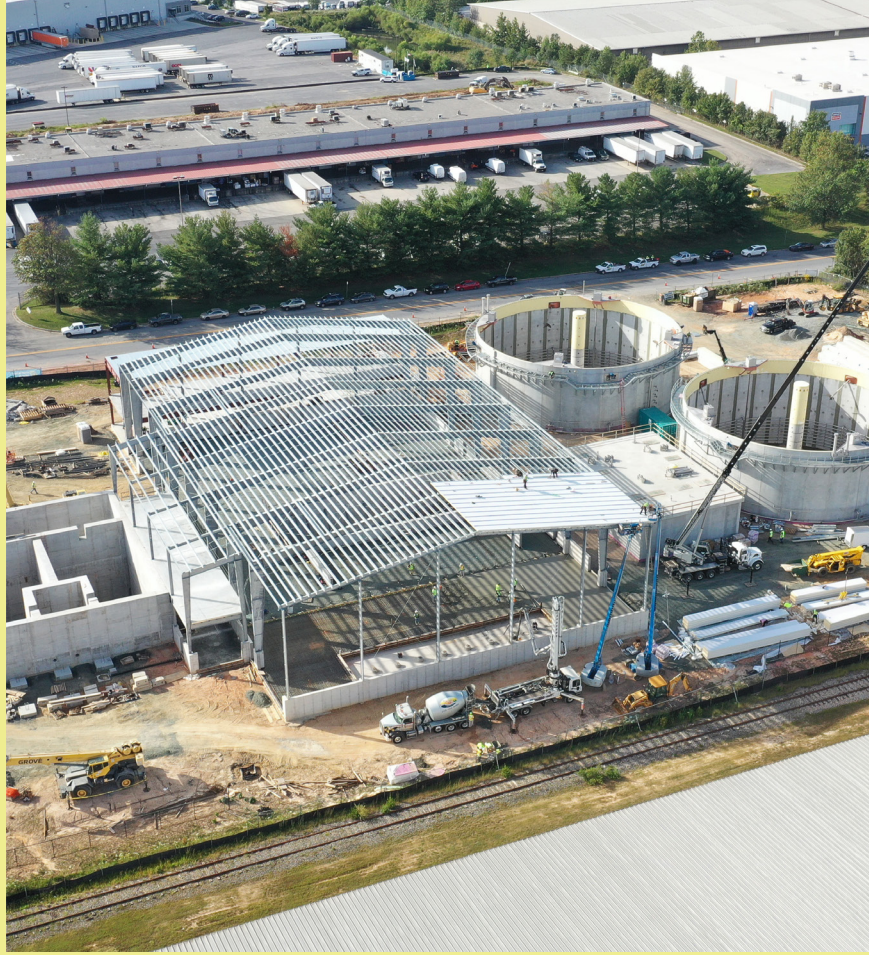
BioEnergy DevCo's food waste digester under construction at the Maryland Food Center Authority in Jessup.
