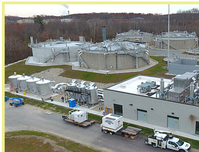
Greater Lawrence Sanitary District (GLSD) anaerobic digesters.
