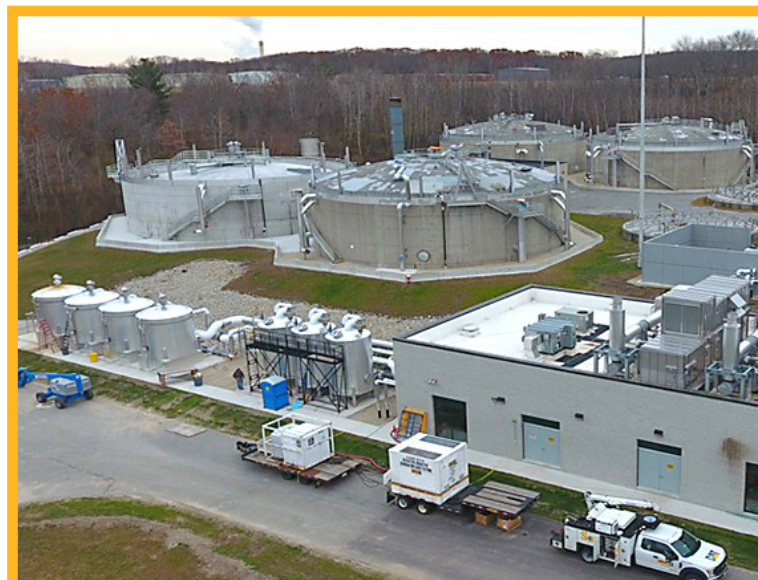
Greater Lawrence Sanitary District (GLSD) anaerobic digesters.
