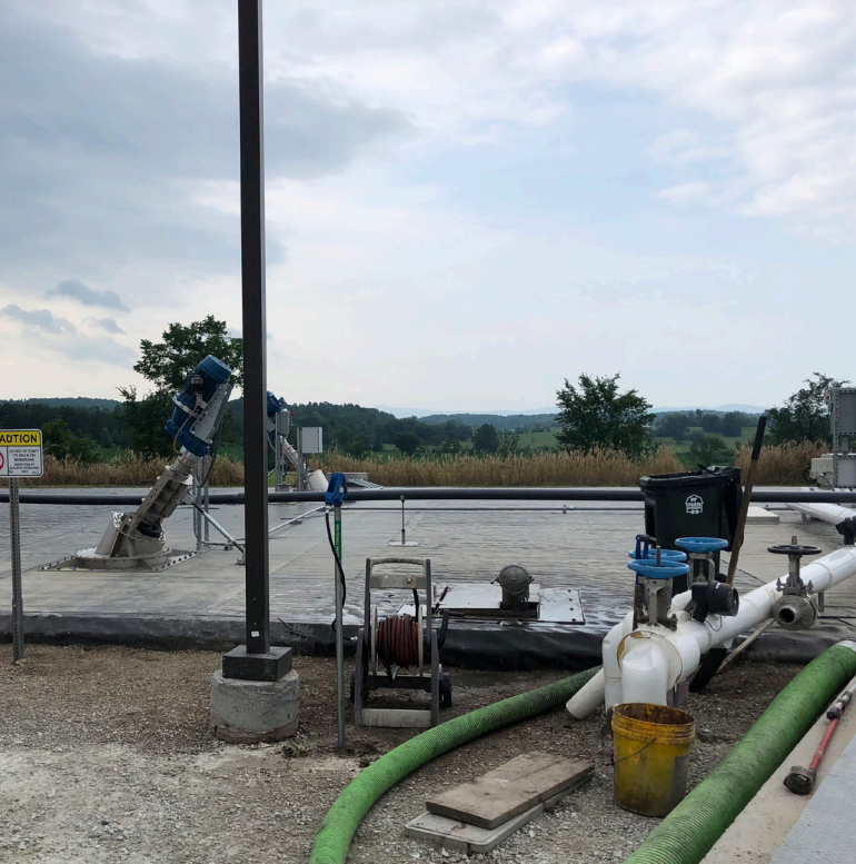
Food waste is unloaded into a hydrolyzer tank at Vermont farm digester in Vanguard Renewables' network.
