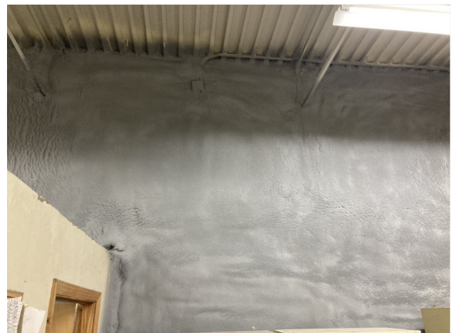
Figure 1. Spray foam insulation installed on interior open wall at Salvation Army, Springfield, MA
